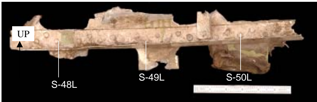
Figure 1.16-105 As received condition of the STA 2160 frame segment submitted for examination. The aft surface is shown in this view.
