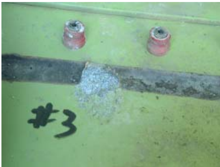
Figure 1.16-136 Higher magnification of #3 corrosion pit, before cleaning (1.56X)
