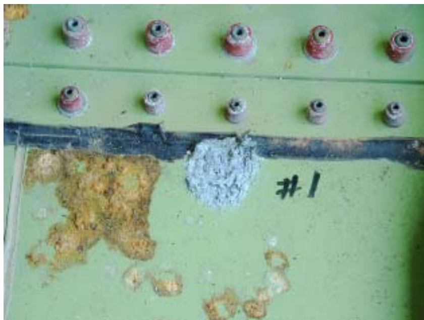
Figure 1.16-134 Higher magnification of #1 corrosion pit, before cleaning (0.71X)
