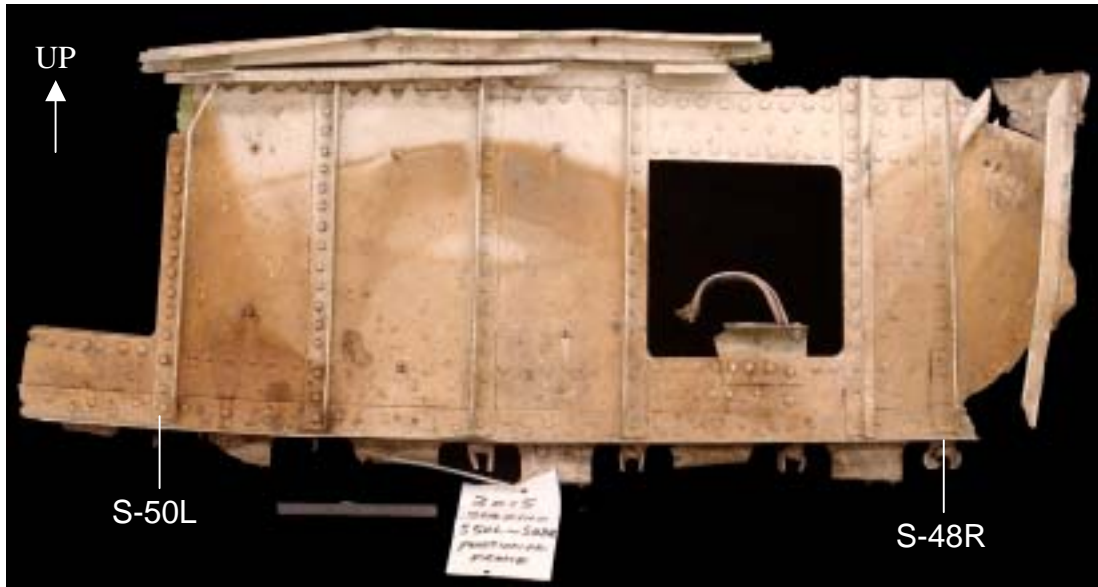
Figure 1.16-109 As received condition of the STA 2100 frame segment submitted for examination. The aft surface is shown in this view.
