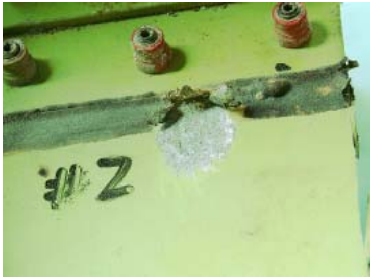
Figure 1.16-140 Higher magnification of #2 corrosion pit, after cleaning (1.40X)
