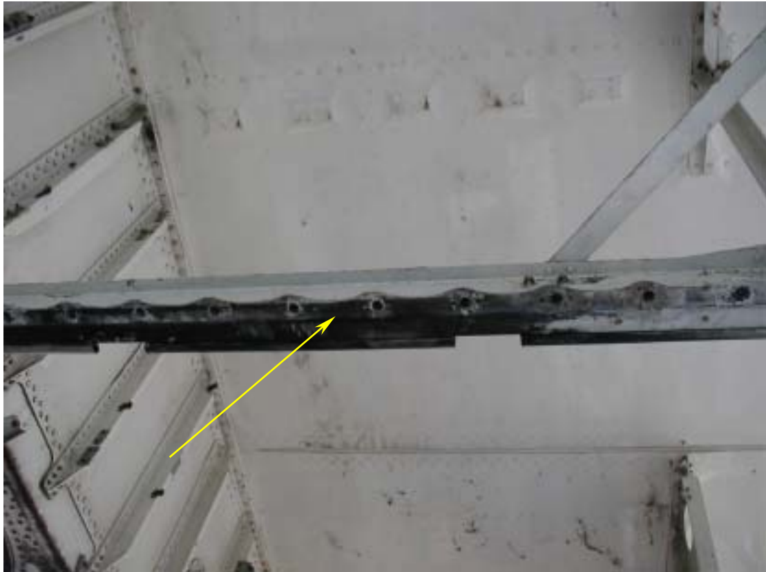
Figure 1.16-175 Photo showing location of sample taken from wing-to-body fairing chord from retired 747
