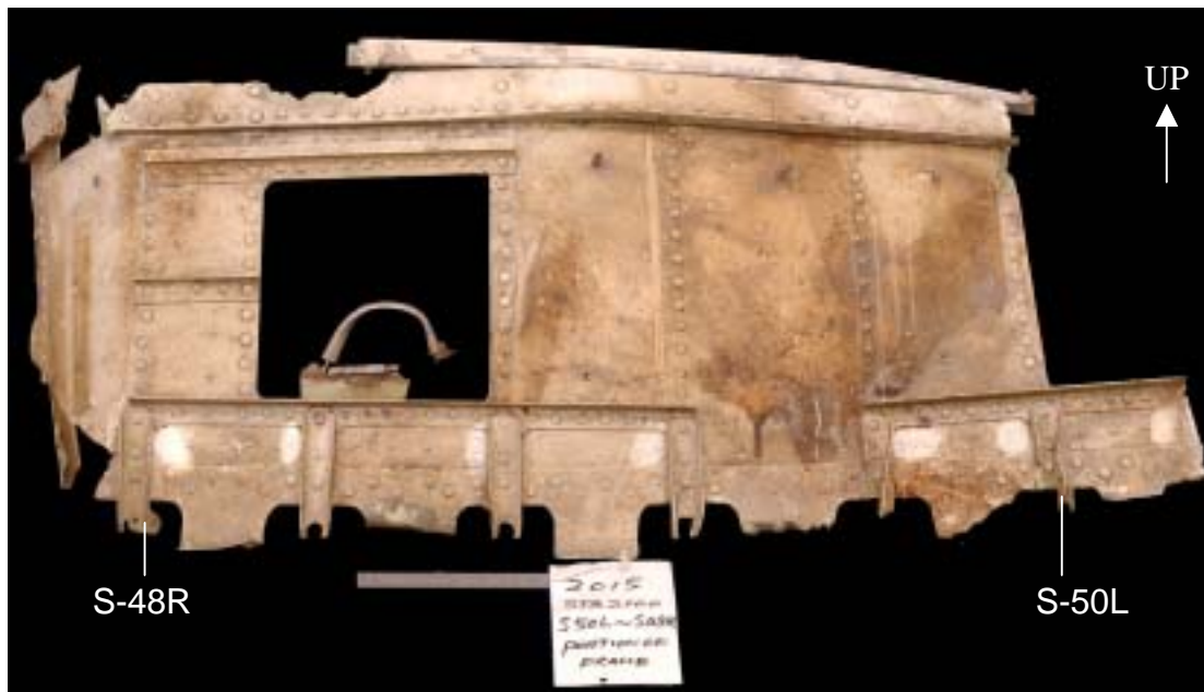
Figure 1.16-110 As received condition of the STA 2100 frame segment submitted for examination. The forward surface is shown in this view.
