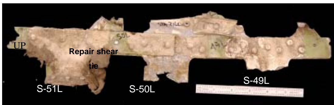
Figure 1.16-106 As received condition of the STA 2160 frame segment submitted for examination. The forward surface is shown in this view.
