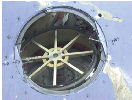
Figure 82: Upper Pressure Relief Valve, close-up showing markings.
