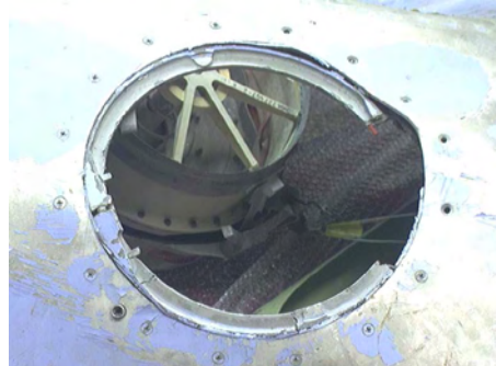
Figure 179: Exterior opening for Lower Pressure Relief Valve (valve still inside).
