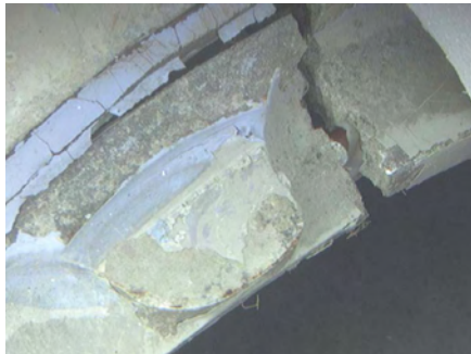
Figure 200: Lower stop pad, with adjacent crack on housing.
