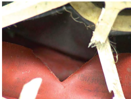
Figure 229 : Outer diaphragm, torn location.
