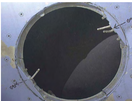
Figure 94: Upper Pressure Relief Valve, pins in approximately "door fully open" position.
