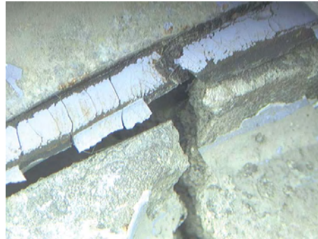
Figure 201: Detail of lower stop pad. • It is broken away from housing (housing cracked).
