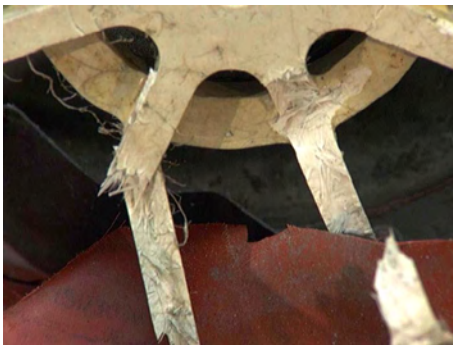
Figure 216: Gate webs, detailed view of broken web members.
