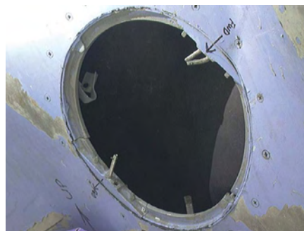
Figure 95: Upper Pressure Relief Valve, same as # 94, another view.
