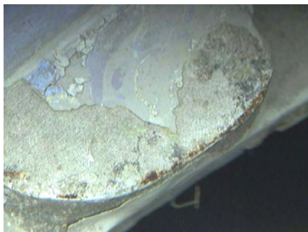
Figure 202: Close-up of figure #200, paint chipped.
