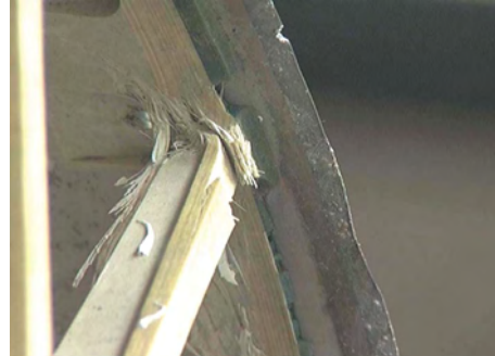
Figure 143: Close-up of web, representative of web fractures at gate ID.
