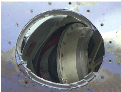
Figure 176: Lower Pressure Relief Valve as viewed from outside, still installed but not attached to structure. (Ref. For following section on pins and stops)
