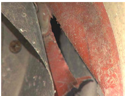
Figure 228 : Outer diaphragm, approximately 60% of circumference is torn.
