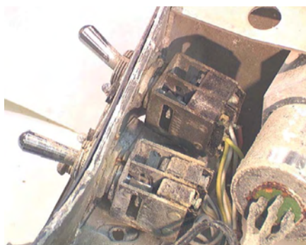
Figure 22: Outflow Valves, MANUAL CONTROL, OPEN & CLOSE toggle switches as viewed from underneath.
