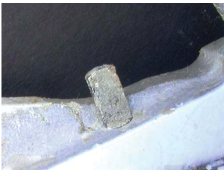
Figure 119 : Overview of forward/upper stop pin, as viewed from outside.
