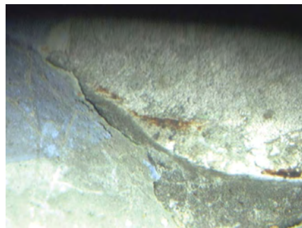
Figure 203: Close-up of figures #200 and #202, slight dent on pad, paint chipped.
