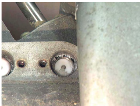
Figure 256: Opposite end of integral sensor poppet and guide; heavy salt deposits.
