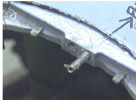
Figure 102: Forward stops and hinge pins, (looking from outside to inside). • Forward/upper hinge pin can rotate freely. • Stop pins look normal and unbent.
