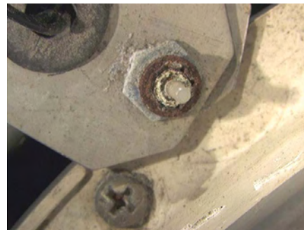
Figure 152: Upper Pressure Relief Valve; valve gate & switch bracket.
