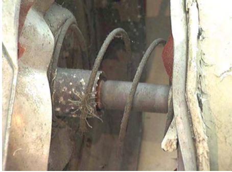
Figure 236: Gate return spring, HS P/N 727414-2 appears to be intact.
