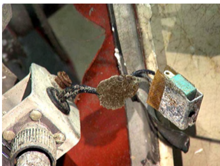
Figure 213: Switch lead wires showing bond detached from housing.
