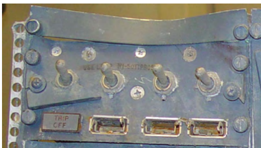
Figure 52: Galley Power control panel M179 • Light plate is missing. • All switch toggles are in up position. • TRIP OFF indicator lights, numbers 2, 3 & 4 legend plates, bulbs and retaining assemblies are missing.
