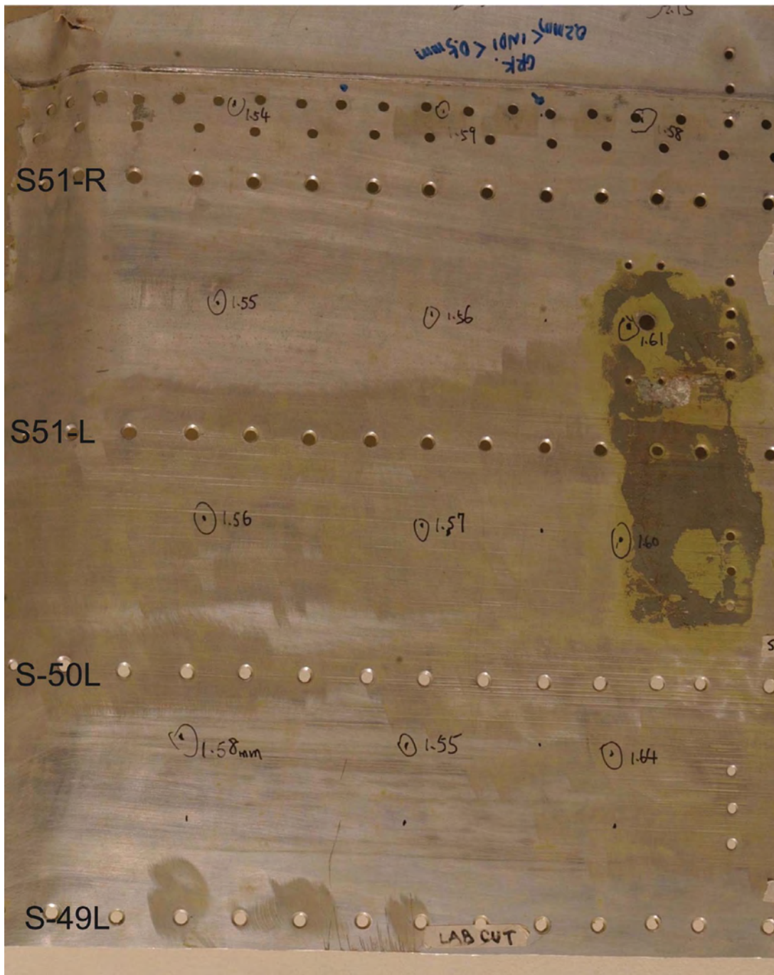
FIGURE 29. EXTENT OF DAMAGE CONSISTENT WITH A TAIL STRIKE – Scratches may be noted at S-50L and S-51L. Scratches may also be noted at the shear tie between S-49L and S-50L.
