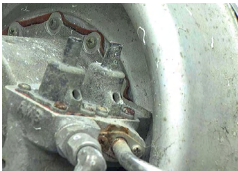
Figure 157: Exterior view of sensors, showing some apparent corrosion on the integral ambient sense tube.
