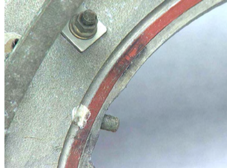
Figure 100: Discolored region of gate seal. • Unknown white colored contaminant on seal.
