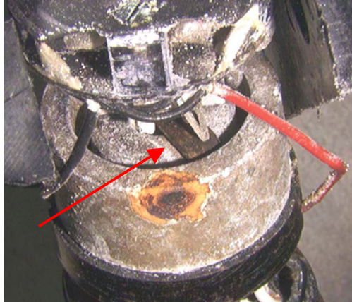
Figure 17: LEFT, OUTFLOW VALVES Position Indicator witness mark
