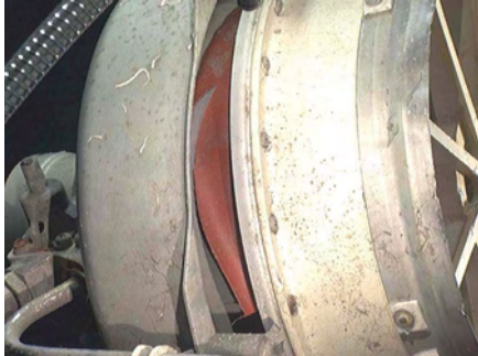
Figure 148: Diaphragm, circumferential tear.
