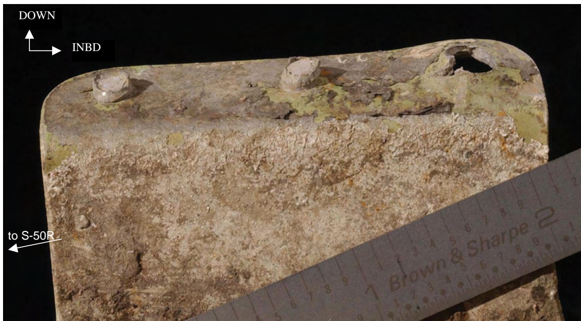
Figure 78. Shear tie between S-51R and S-50R of the STA 2100 frame segment showing downward deformation in skin flange and pull through of the fastener hole at the inboard most fastener hole.
