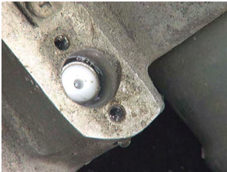
Figure 169: Shows water in plug area.
