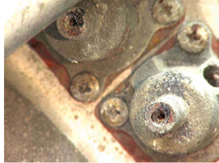
Figure 242: Control adjustment screws, both appear to be intact.
