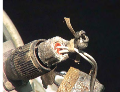
Figure 210: Electrical switch connector interface appears to be intact. • Wires are intact exiting plug. • Strain relief on backshell is broken.
