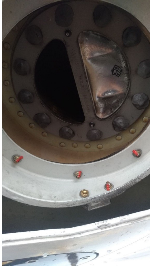
Figure 1.6-1 Failure Position of the Ground Connection Check Value
