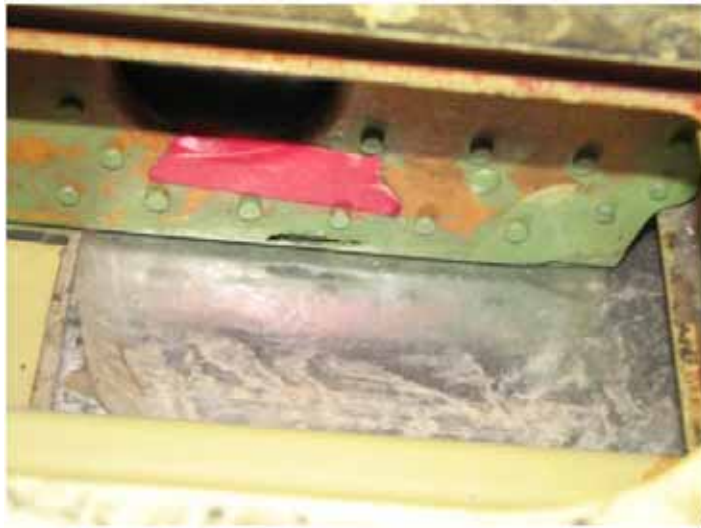
Figure 1.12-49 Corroded Intercostal with Material Lost Through Hole
