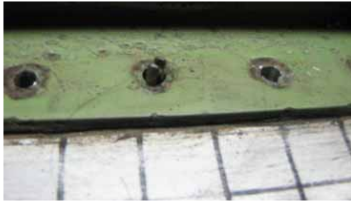
Figure 1.12-30 Deep Corrosion in G5 Area
