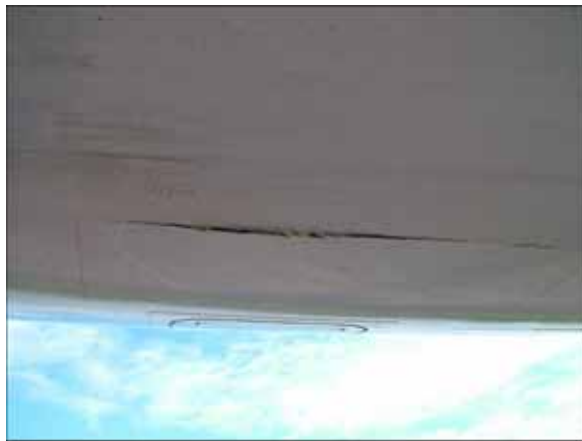
Figure 1.12-1 (B) Location of Crack
