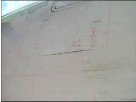
Figure 1.12-1 (A) Cracked Skin External View
