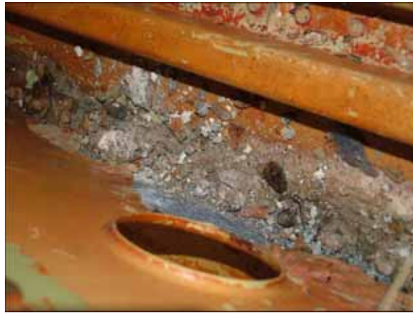
Figure 1.12-2 (S) The Corroded Intercostal Close up View
