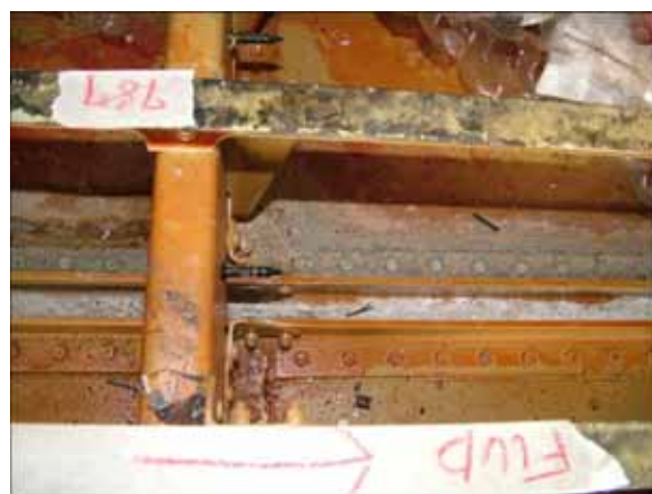
Figure 1.12-2 (B) Corrosion forward of Sta. 78
