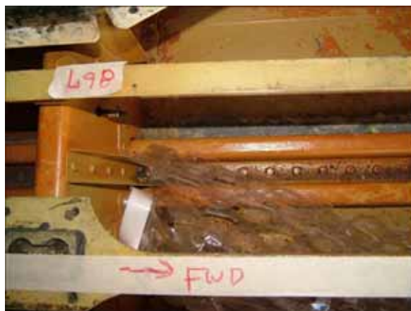
Figure 1.12-2 (O) Corrosion forward of Sta. 867
