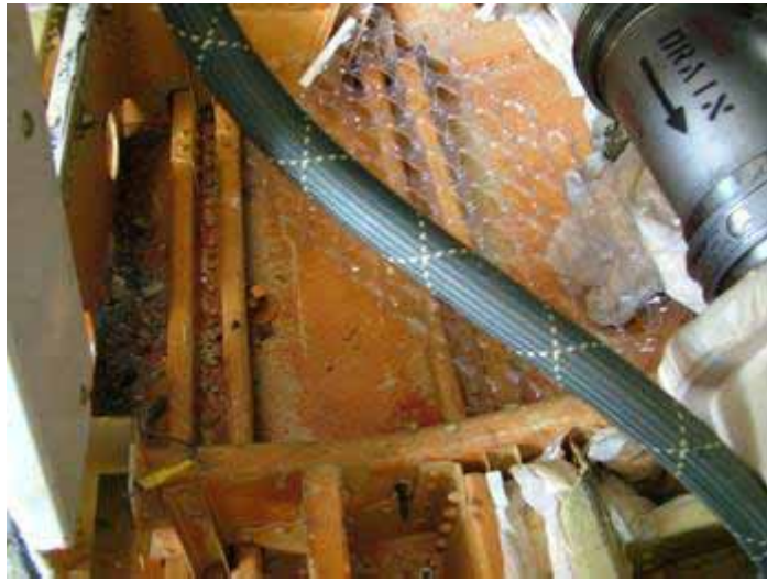
Figure 1.12-51 Leakage Downstream to Corroded Intercostal
