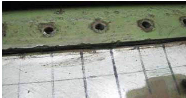
Figure 1.12-28 Deep Corrosion Found in G3 Area
