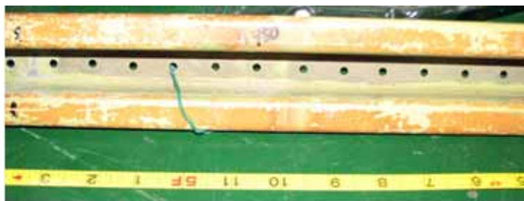
Figure 1.12-45 BS 947~BS 956 Corrosion with G15 Area
