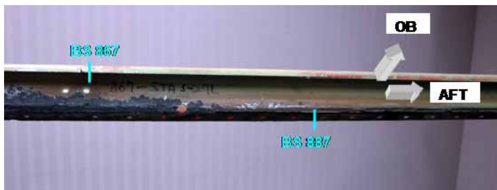
Figure 1.12-40 Corrosion Area G12-B
