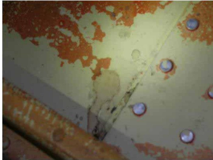
Figure 1.12-7 Leakage Trace over The Skin Panel
