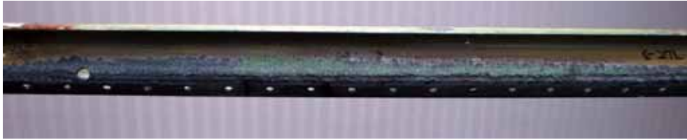
Figure 1.12-36 Corrosion in G10-B Area
