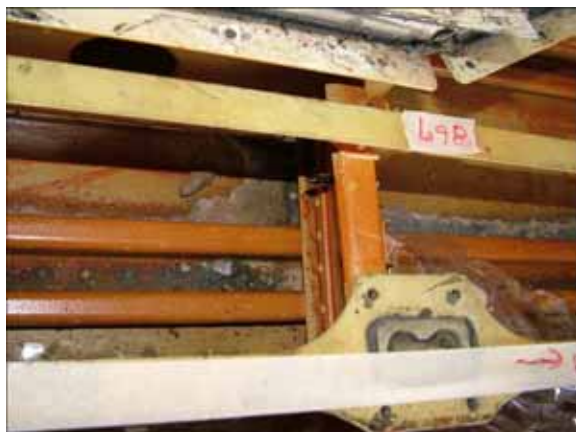
Figure 1.12-2 (P) Corrosion aft of Sta. 867
