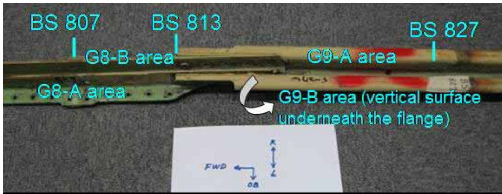
Figure 1.12-33 Corrosion Sites G8-A, G8-B, G9-A, G9-B
