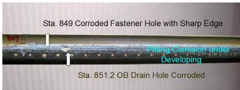
Figure 1.12-38 Corrosion Area G11-B
