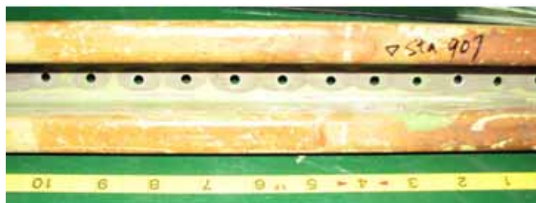
Figure 1.12-42 BS 907~BS 917 Corrosion with G13 Area
