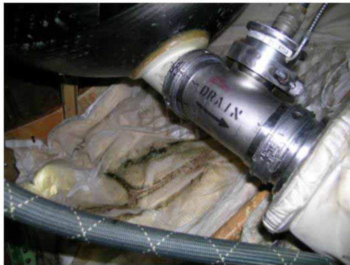
Figure 1.12-5 Trace of Contamination from Leaked Waste Water
