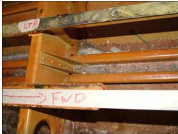
Figure 1.12-2 (L) Corrosion forward of Sta. 847
