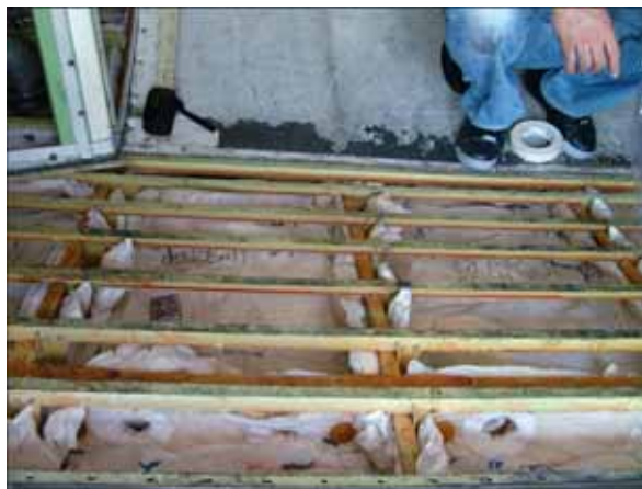
Figure 1.12-2 (A) Floor panel Open Up Inspection for Skin Damage
