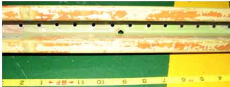
Figure 1.12-48 Corrosion Area G17
