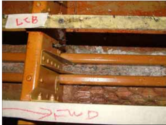
Figure 1.12-2 (I) Corrosion forward of Sta. 827
