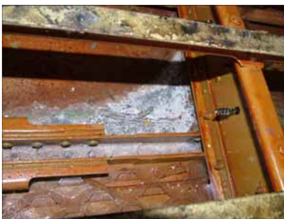
Figure 1.12-2 (H) Skin Corrosion aft of Sta. 807 Close up View
