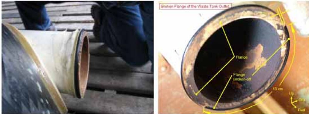
Figure 1.12-9 Damage of the Waste Tank Outlet Port
