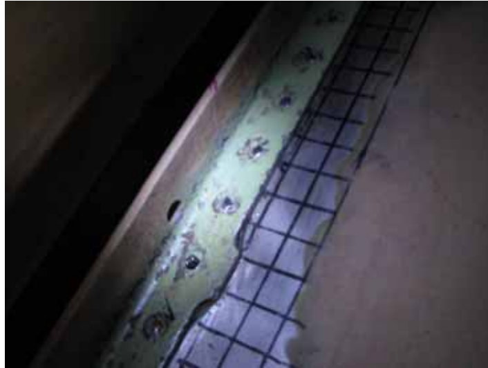
Figure 1.12-32 Deep Corrosion in G7 Area
