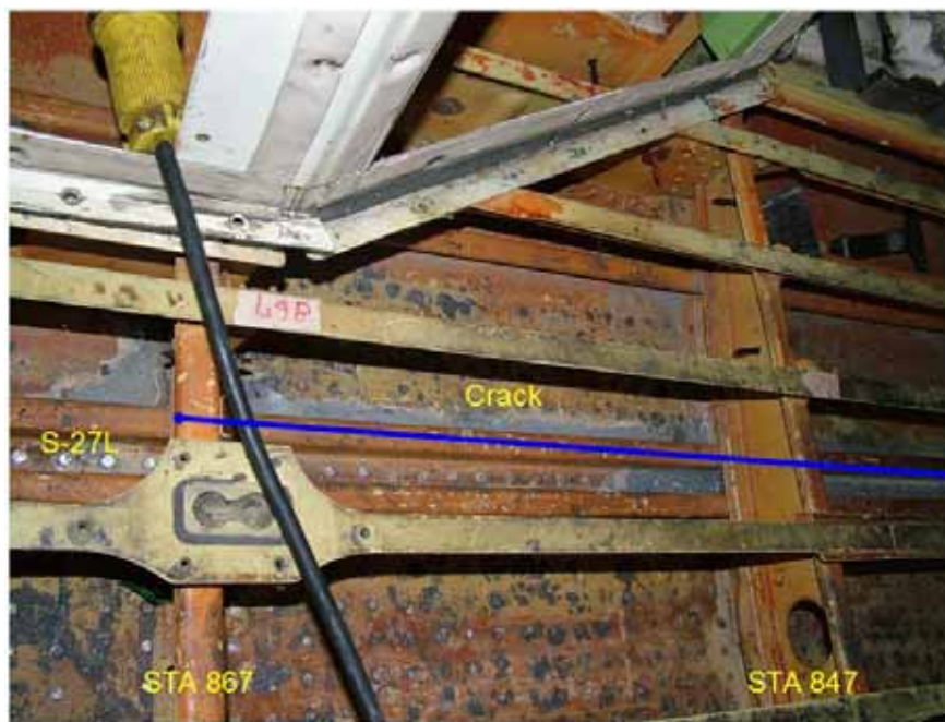
Figure 1.16-3 Location of crack adjacent to the S-27L stringer
