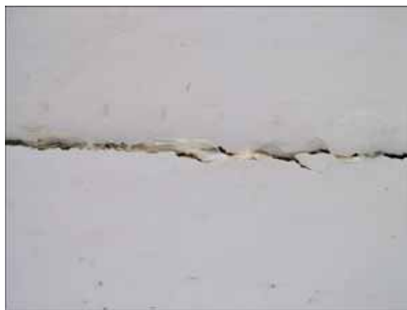
Figure 1.12-1 (C) Detail Cracked Skin External View
