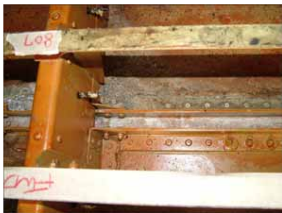
Figure 1.12-2 (E) Corrosion forward of Sta. 807 Close up View
