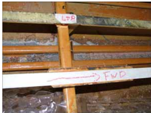
Figure 1.12-2 (K) Corrosion at Sta. 847
