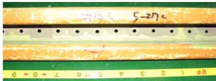
Figure 1.12-43 BS 917~BS 927 Corrosion with G13 Area
