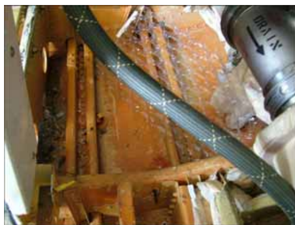
Figure 1.12-2 (Q) Relative Position of the Leaking Waste Tank Outlet and the Corroded Intercostal
