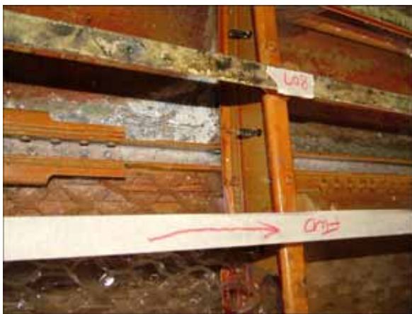
Figure 1.12-2 (G) Skin Corrosion aft of Sta. 807
