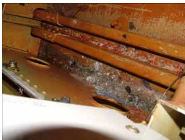
Figure 1.12-2 (R) The Corroded Intercostal
