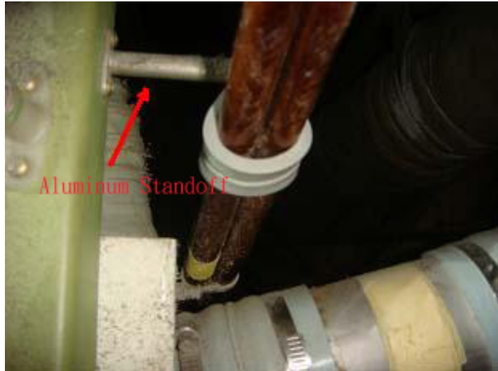
Fig. 1.6-1 Fixture of APU Generator Wires
