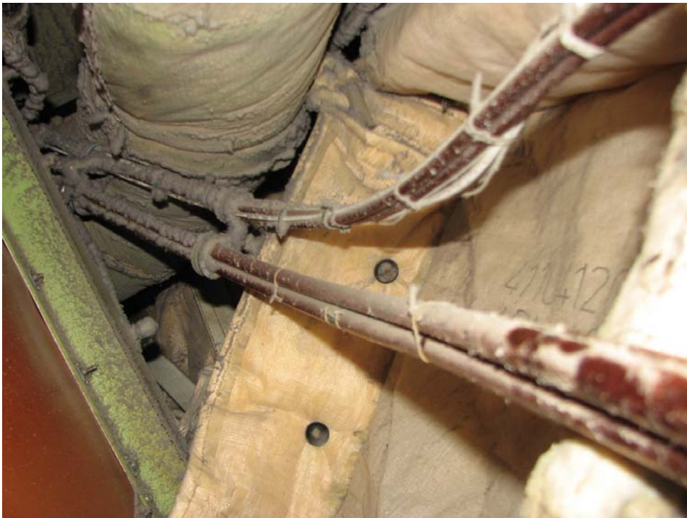
Fig. 1.12-14 Dust on Other System Components
