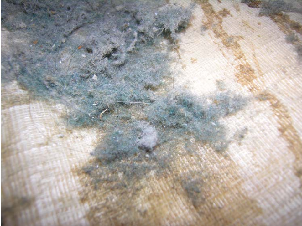
Fig. 1.12-18 Close up View of the Contamination on Insulation Blanket
