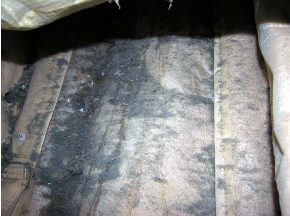
Fig. 1.12-13 Dust and Traces of Contamination on Insulation Blanket
