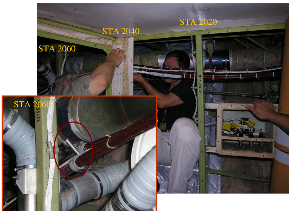
Fig. 1.12-22 The Relative Position of The Damaged Standoff to Fuselage Structure
