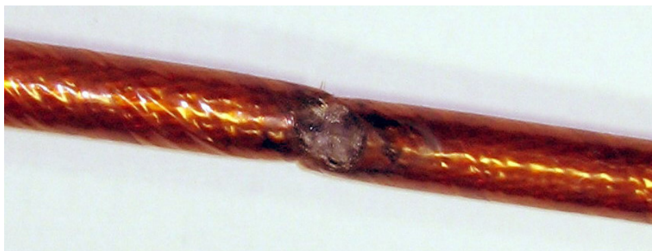
Fig. 1.12-20 APU Power Cable with Damaged Insulation Jacket
