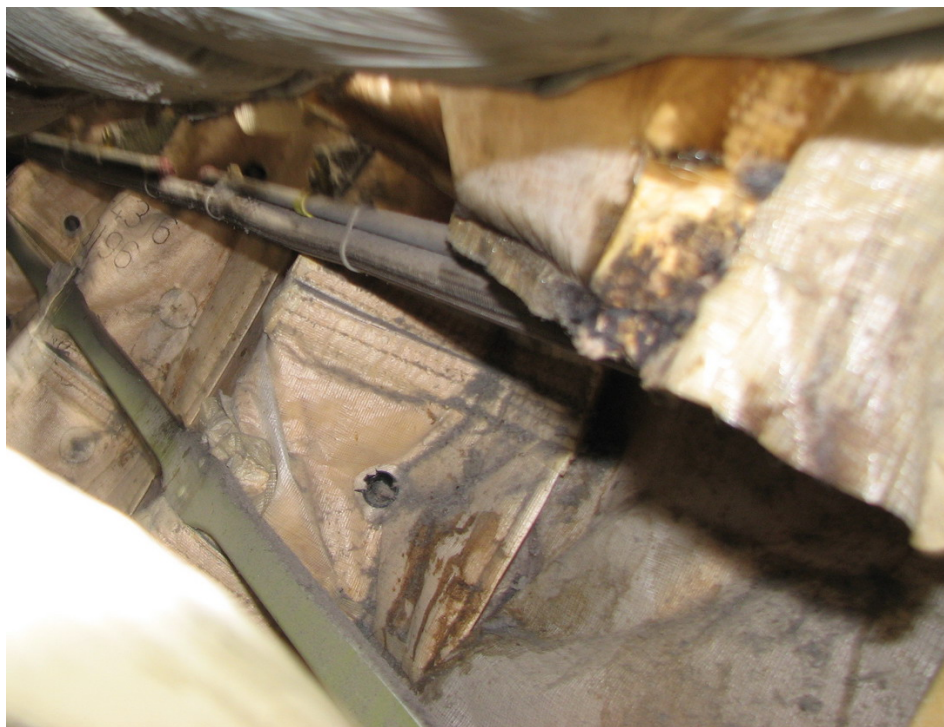
Fig. 1.12-12 Dust and Traces of Contamination on Insulation Blanket
