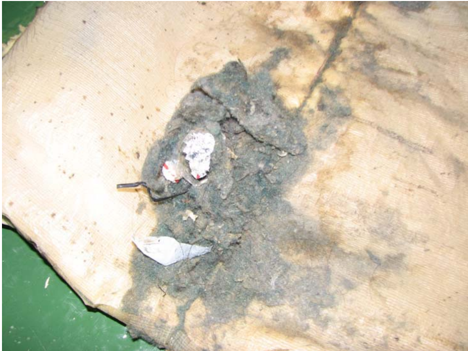
Fig. 1.12-11 Contamination, Dust and Cabin Items on the Damaged Insulation Blanket
