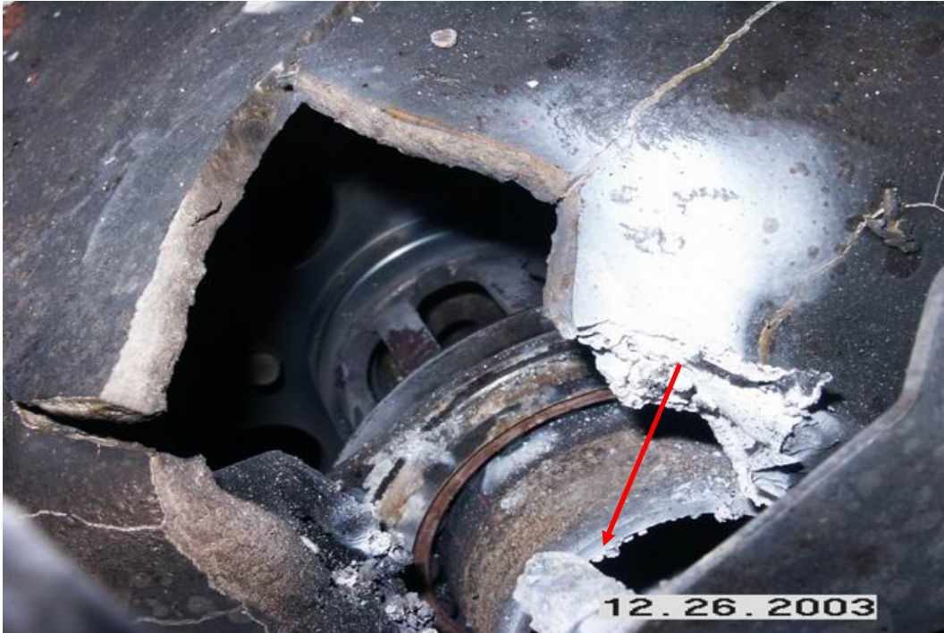
Figure 2.3-2 Severe wear in brown coloration on the outer diameter of impeller shaft (red arrow); stains of white ashes around the fractured area of rear inlet case.
